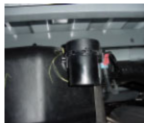
Figure C1, Step 1: Locate the Fuel Valve.
